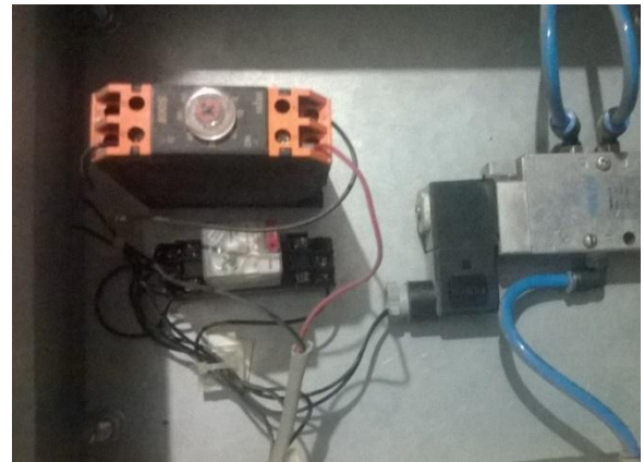
Fig: 7 Circuit board of controller with solenoid and Delay timer
